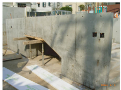
Wall surface waterproofing work for steel reinforcement steel bar block made residential building
